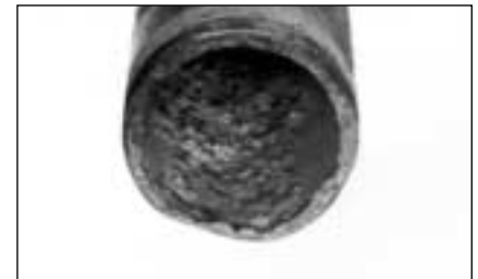
Figure CG-10. Oxygen in the system speeds corrosion (oxidation) of pipes, causing pitting such as shown here.
